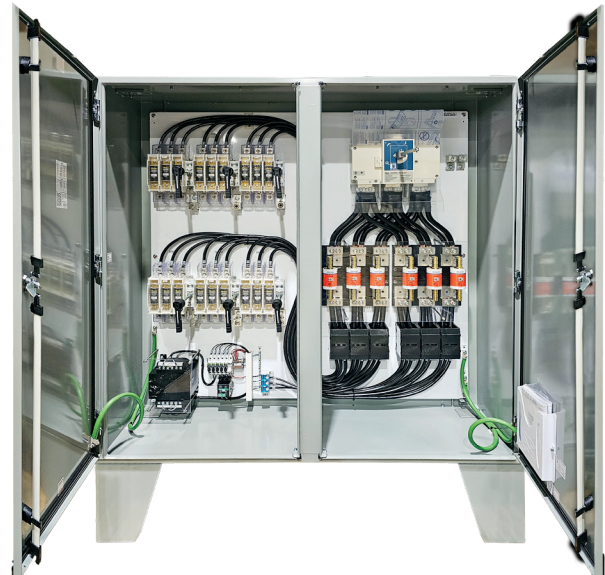
Figure 17: Bank Breaker Panel
